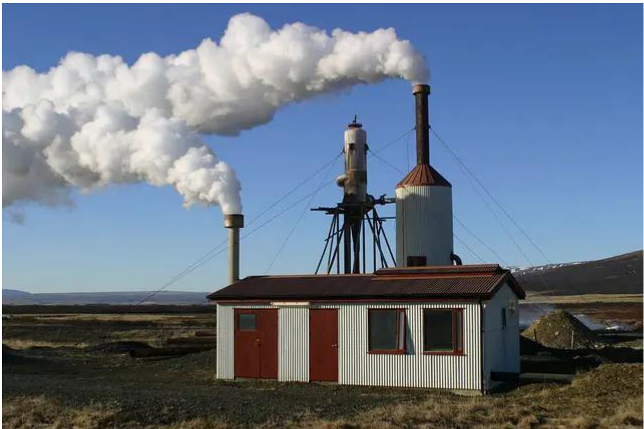
Geothermal Setup In Iceland
